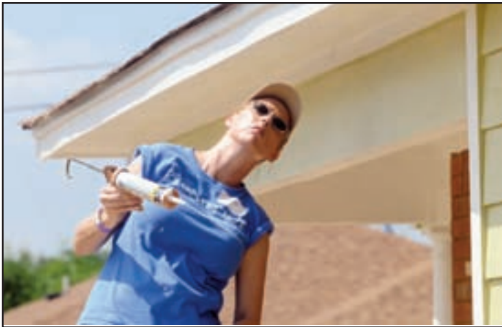
Carolyn Hicks Fry, director of information systems for Baptist Memorial Health Care and Baptist's volunteer coordinator for the Habitat for Humanity build, puts some finishing touches on the outside of the Baptist-sponsored Habitat house.
