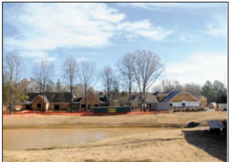
The Baptist Trinity Hospice House and Kemmons Wilson Center for Good Grief construction continues on the campus of Baptist Memorial Hospital-Collierville on Friday, Dec. 11, 2009. The house is scheduled to open in the summer of 2010 and will be the first residential hospice house of its kind in the area.
