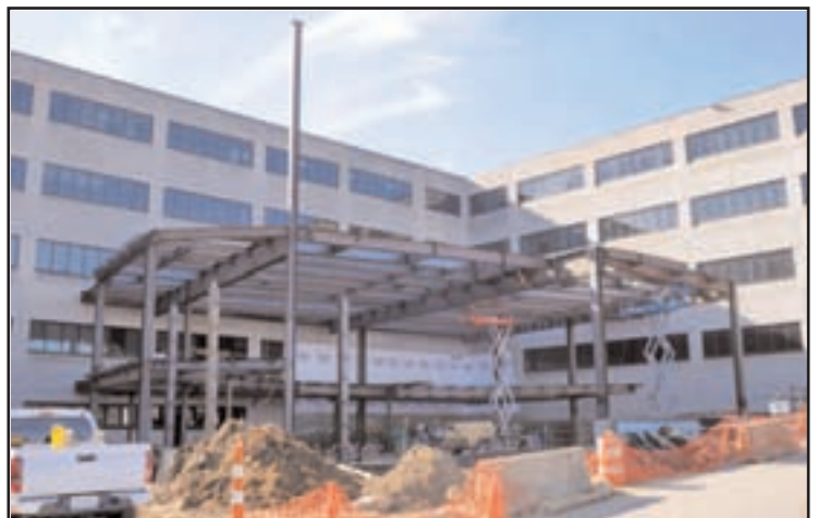
Construction on the Baptist Memphis Education Center and Dr. H. Edward Garrett Sr. Auditorium continues on Friday, Dec. 11, 2009. The center will measure 20,000 square feet and include classroom space and the 282-seat Garrett Auditorium, named for one of the men who performed the first successful open-heart surgery 45 years ago. A donation from the late Dr. Garrett's family helped make the new center and auditorium possible.
